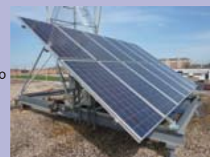
Typical Suns Strut Photo Voltaic Installation
